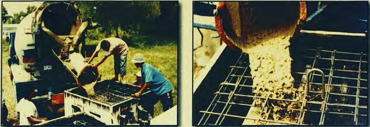
Figure 11 : A ready-made cement mixture with the mixture ratio of 3:1.5:1 for sand, gravel and cement
