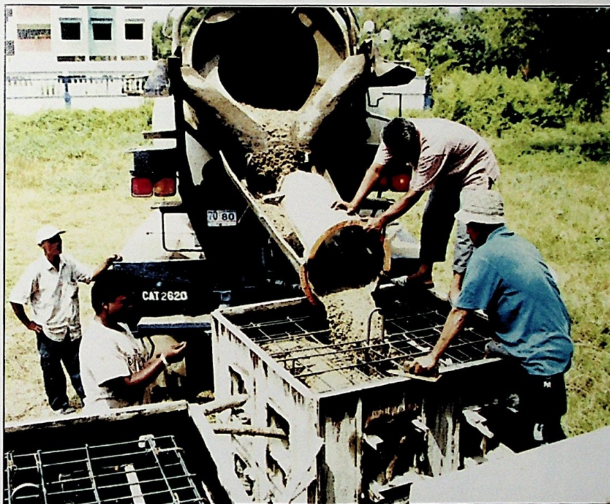
Figure 11 : A ready-made cement mixture with the mixture ratio of 3:1.5:1 for sand, gravel and cement
