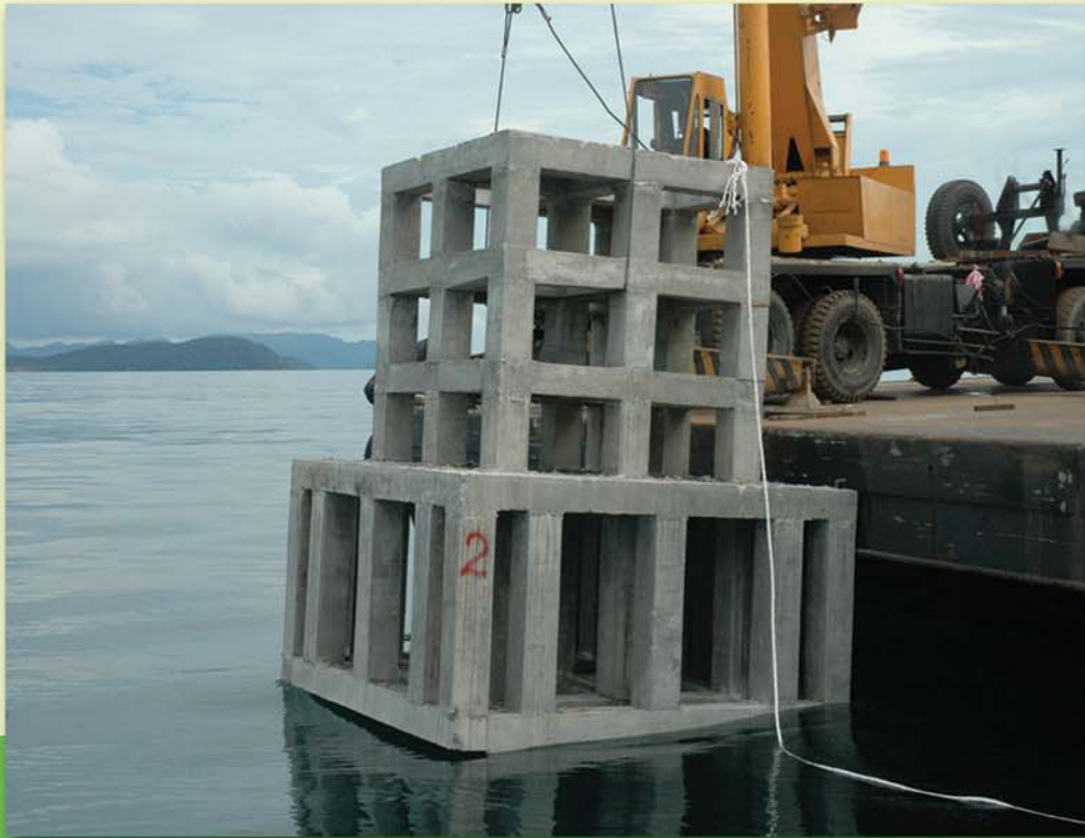
Deployment of artificial reef for soft bottom at Kuala Teriang, Langkawi, Kedah.
